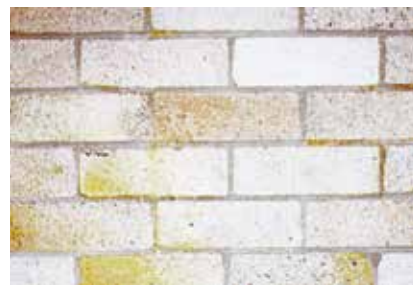
Figures 9 & 10. Iron stains
