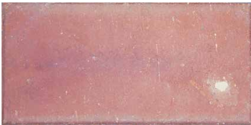
Figure 7. Example of lime pitting
