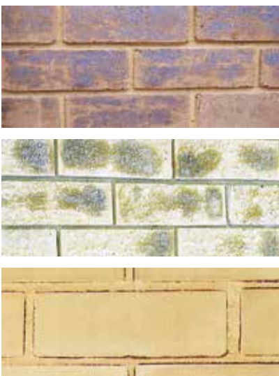
Figures 11, 12 & 13. Manganese stains
