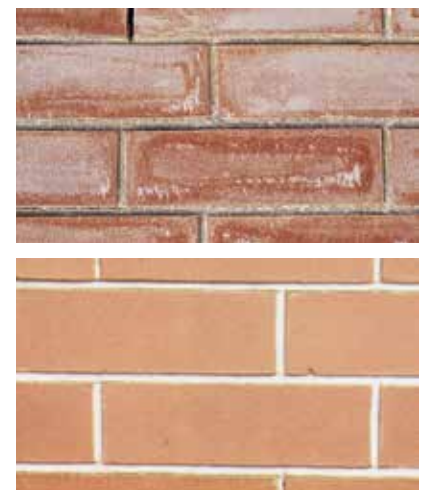
Figures 16 & 17. Efflorescence before and after cleaning
